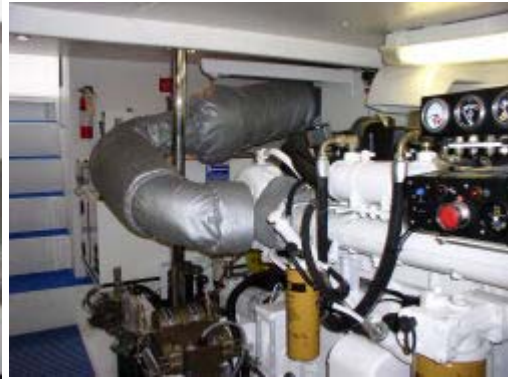
Engine Room to Port
